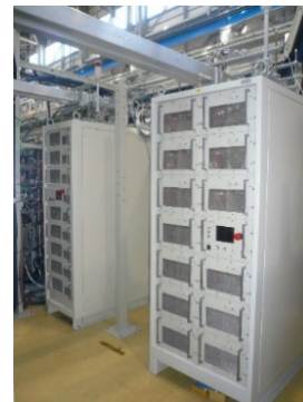
Figure 2: RF power sources in ML: 16 kW (right) and 8 kW (left) SSAs.
