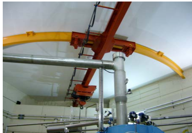
Radial 6-ton crane
