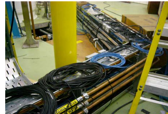
Cabling & Cooling water pipes
