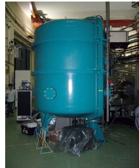
500kV Power Supply
