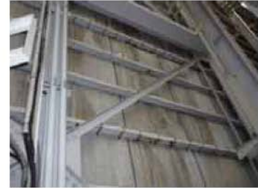
[外壁漏水状況 2]
